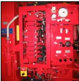
Main control valve cabinet with local control panel. Main control valve cover removed.
